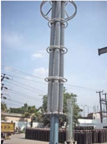
1200KV Lightning Arrester
