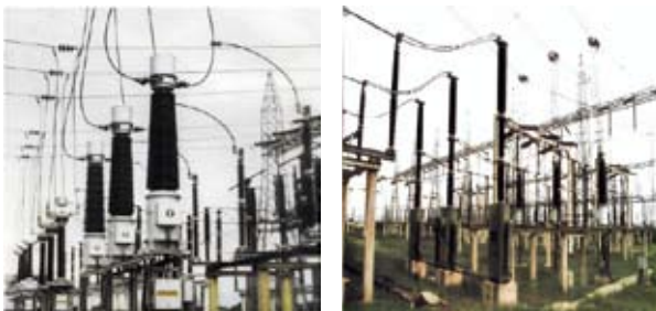
Typical sub-station depicting use of hollow insulators for equipments
