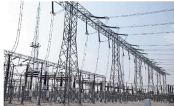
Typical 400 kV sub-station where Disc, Tubular and Solidcore Insulators are used
