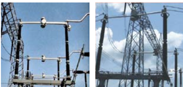
Solid Core Insulators in 400kv switchyard
