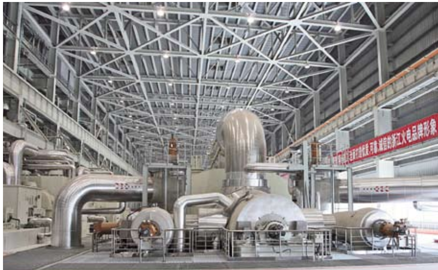
Steam turbine at Yuhuan coal-fired power plant
